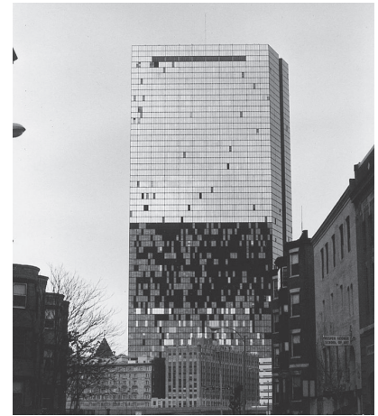
Photo 1.1: Wind damage. Shortly after thermopane windows were installed in this high-rise office building, they began failing and falling out, scattering broken glass on passers-by beneath.
